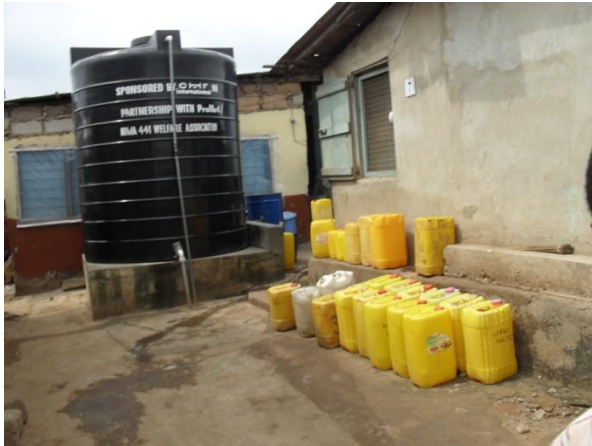
Fig. 2: Large water storage facility obtained through microfinance
