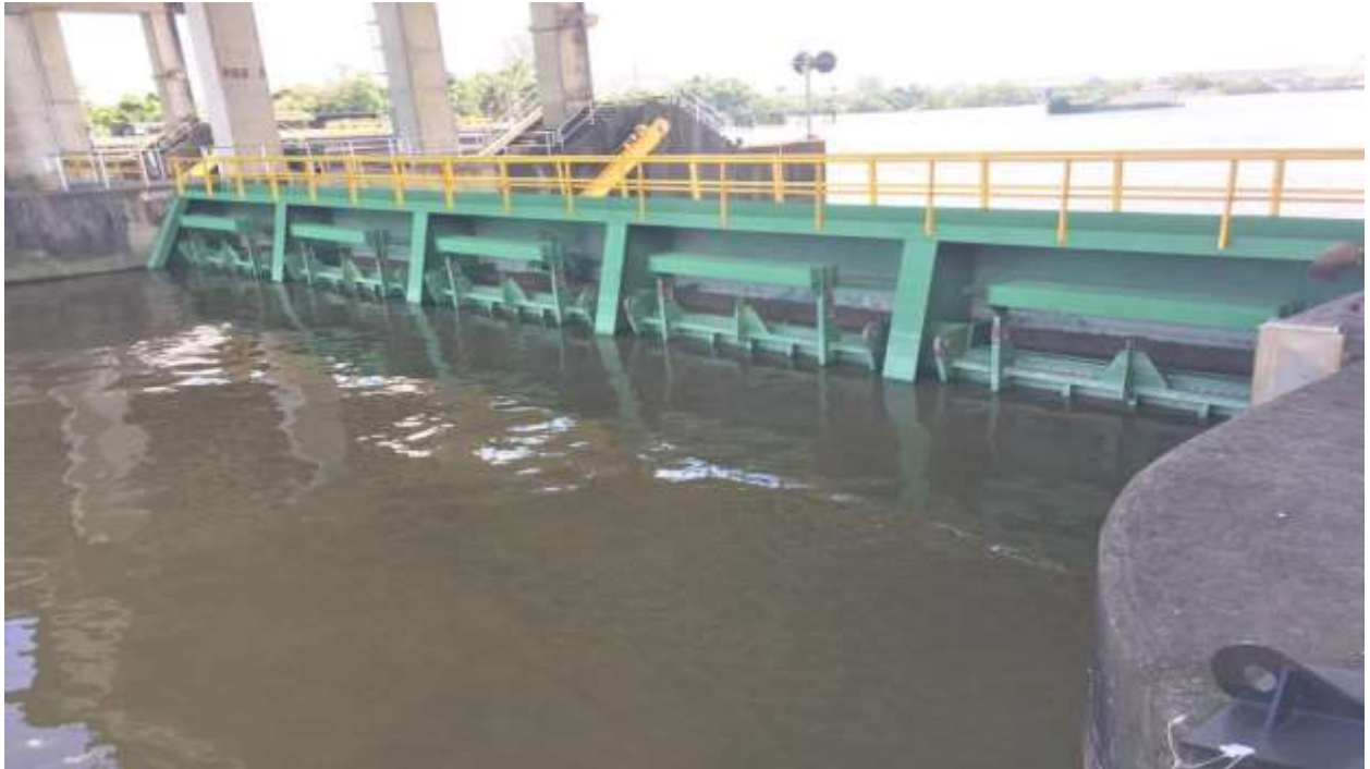
Figure 4: Downriver view of barrage gate 4 spillway flap gates closed when water level downriver is higher than upriver
