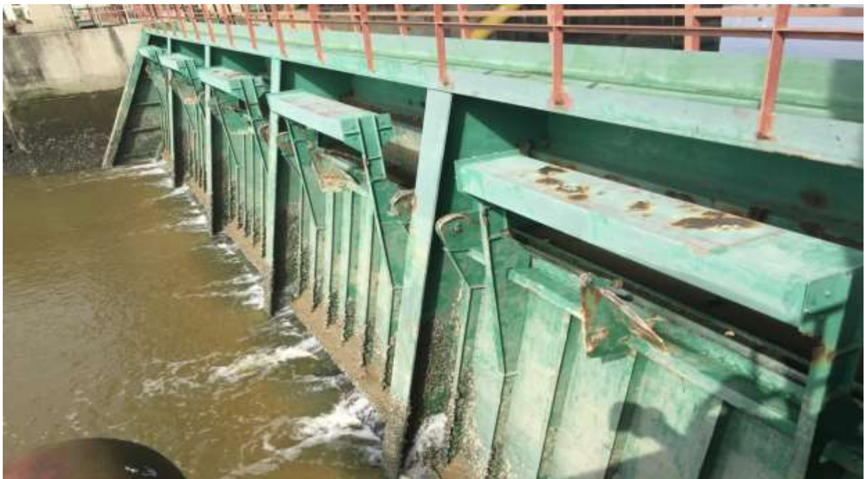
Figure 5: Spillway flap gates locked - pressure from upriver leaking seals taken from downriver
