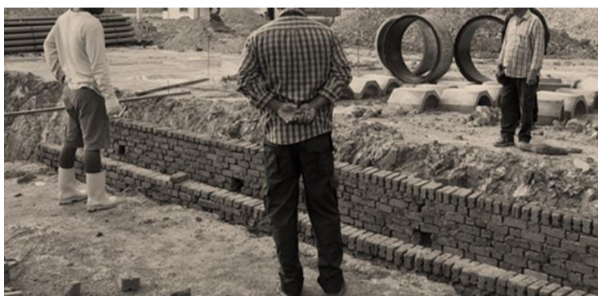
Figure 6. Workers and site workers were discussing about the wrong type of drain built
