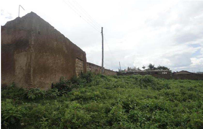
Plate 4 Destroyed shops in Lugari Sub-County
