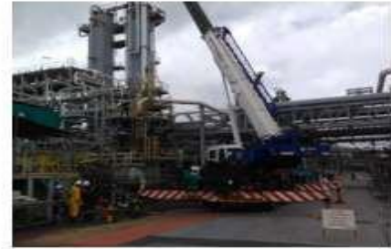
Critical lifting activity over live line with load more than 1tonne
