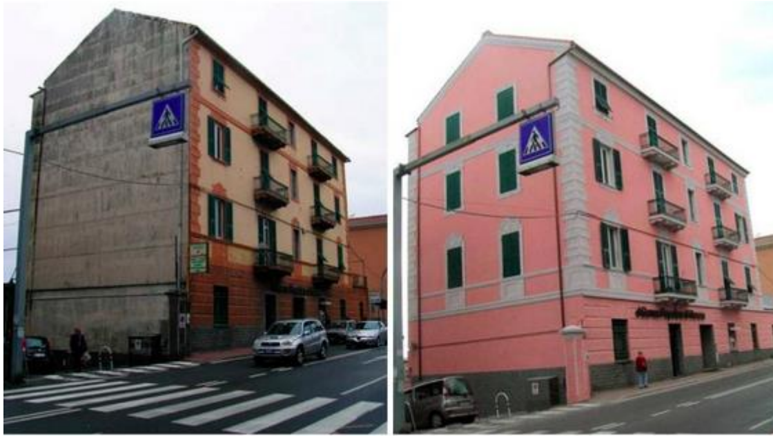
Figure 1: Illustration of a private building in Italy, showcasing its condition before and after undergoing retrofitting in accordance with the EGD EU Directive 2018/844 (Source: https://www.ssorgey.top/products.aspx?cname=cappotto+termico+condominio+prima+e+dopo&cid=56 )
