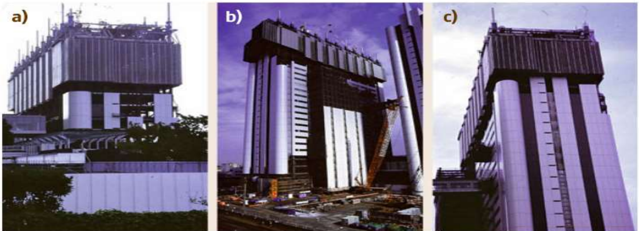
Figure 5 Obayashi Automated Building Construction System (ABCS) (a) early construction phase; (b) intermediate construction phase; (c) final construction phase adopted from (Saidi et al., 2016)
